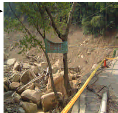
Fig 13. A GIS hyperlinked picture - a damaged reinforced wall
